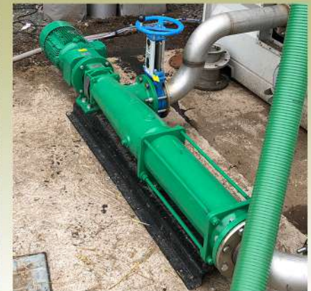
BIOMASS TRANSFER PUMP
