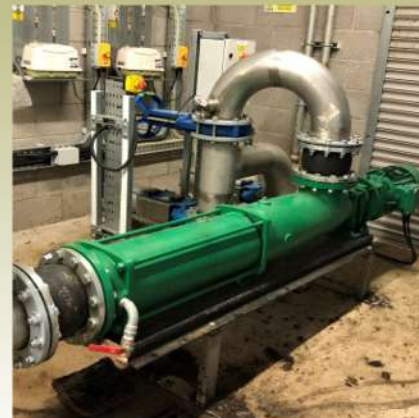
BIOMASS RECIRCULATION PUMP
