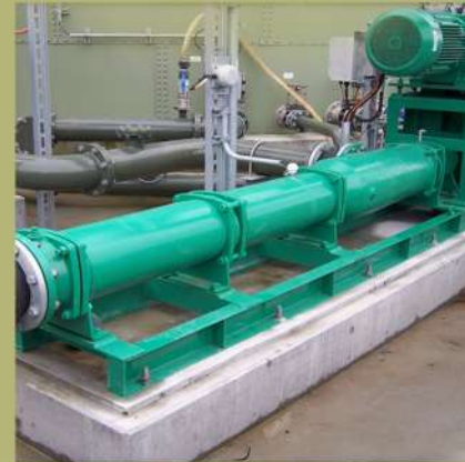
DIGESTATE TRANSFER PUMP
